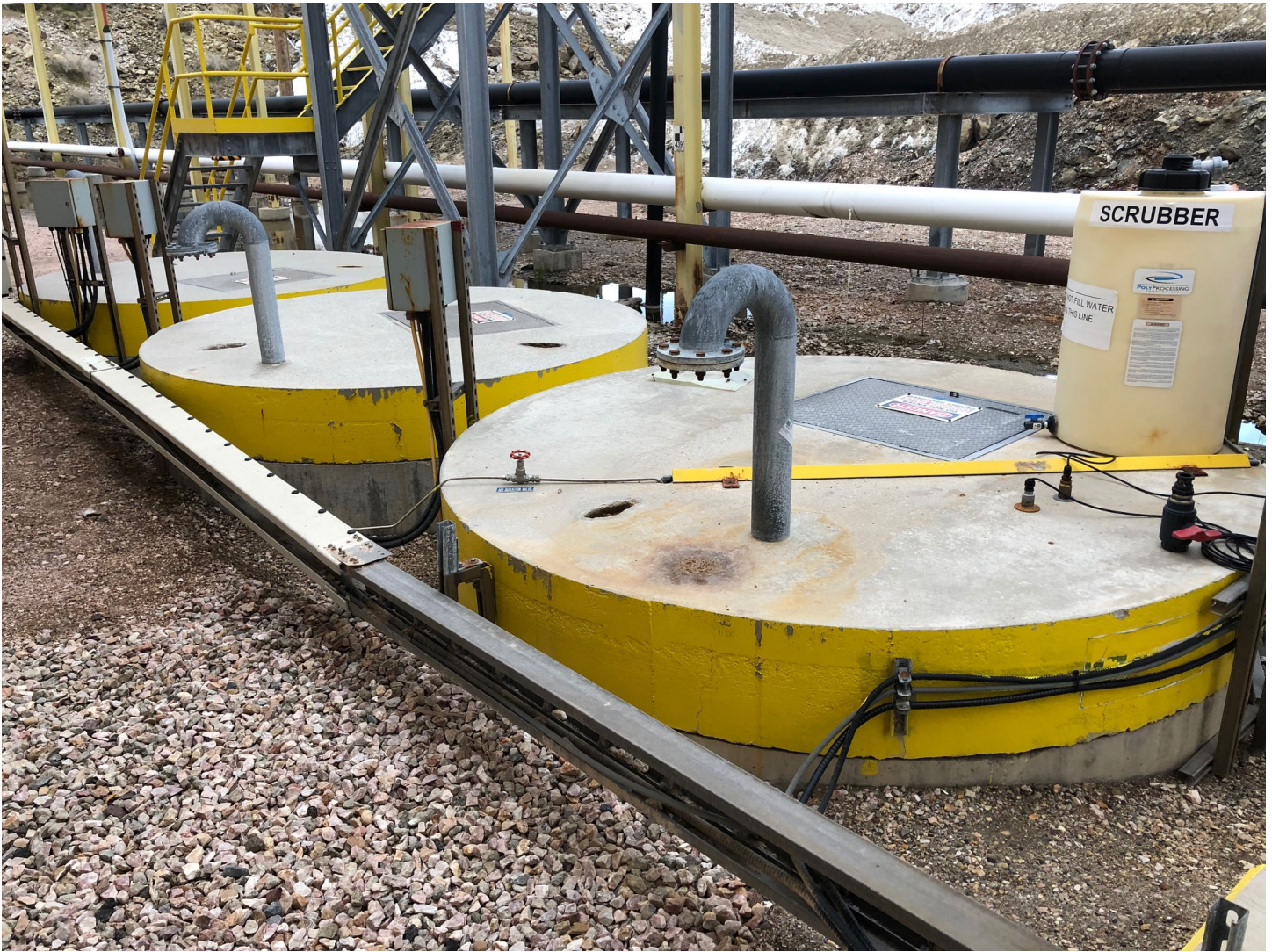
Figure 2 Effluent storage vaults
