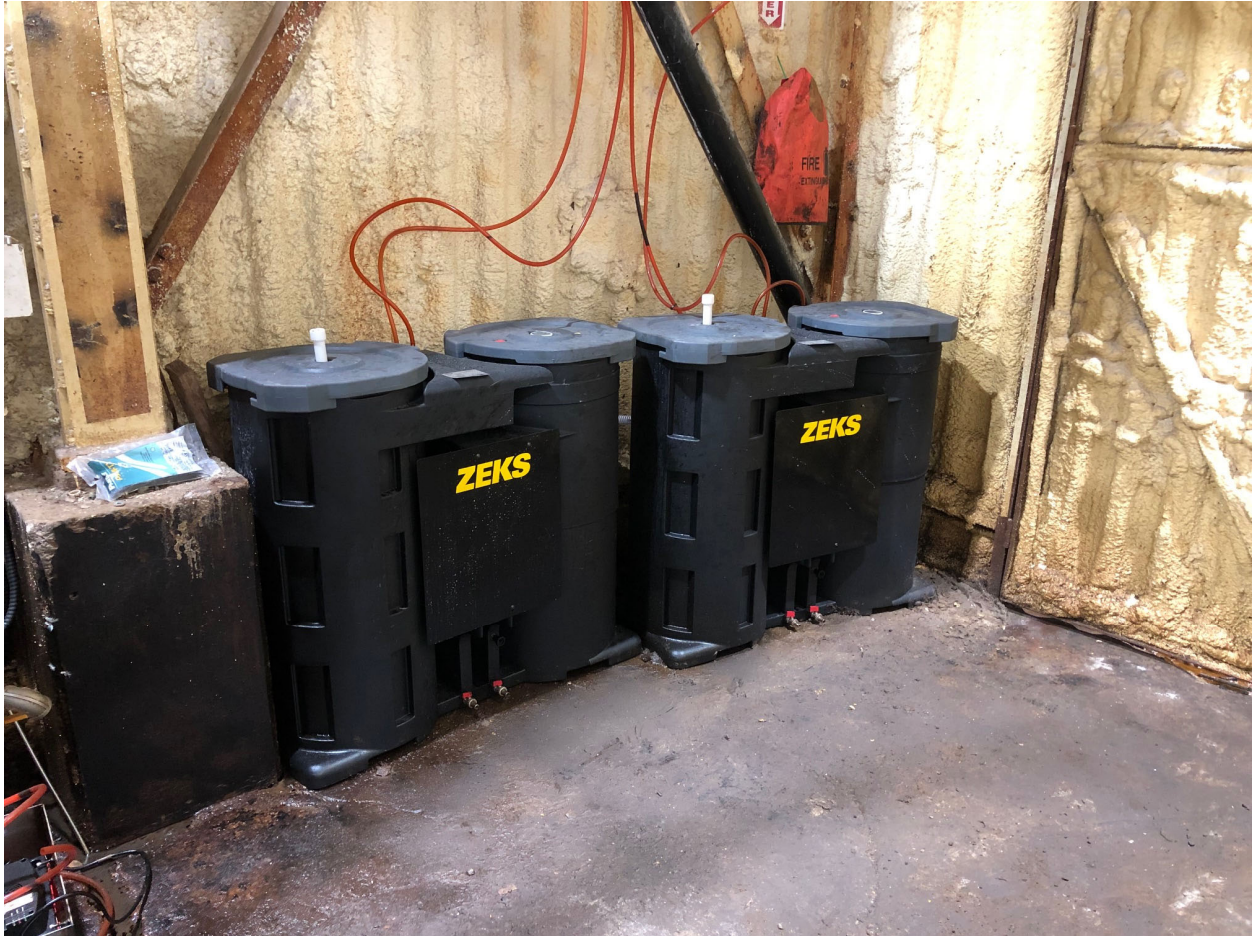
Figure 1 Installed oil/water separators
