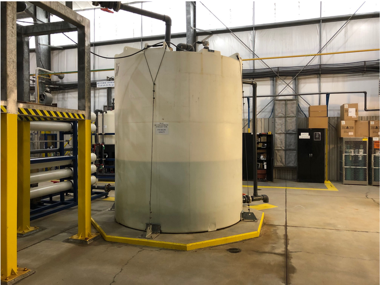
Figure 1 RO concentrate tank
